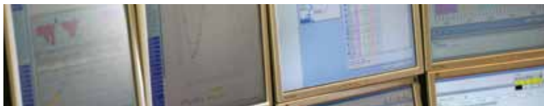
CENTRALISED REMOTE CONTROL OF CNR'S DEVELOPMENT SCHEMES
